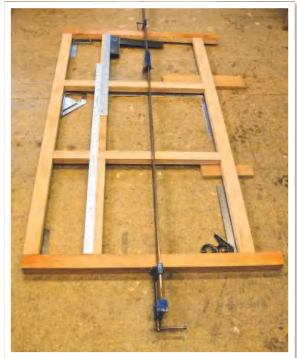
▲ Pic.3 Checking dimensions on a multi-part frame, diagonals checked and all corners square, then the five-part mid rail can be measured using butted metal rules to extend a 1m rule to 1.6m
